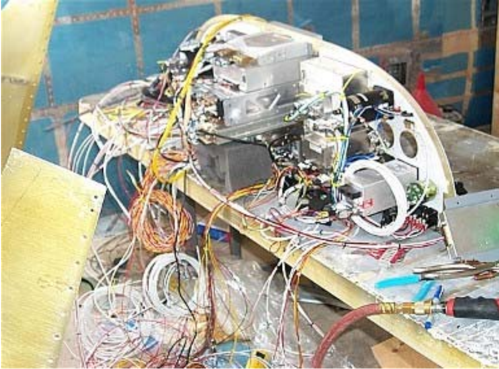
Anybody know where all these wires go.
